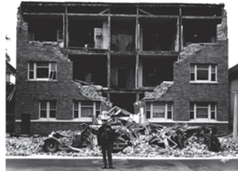
Figure 2 Morrison Apartments, 915 E. Ocean, Long Beach, California 1933 – Front wall only fell away from floors and roof onto street below due to directional properties of earthquake
