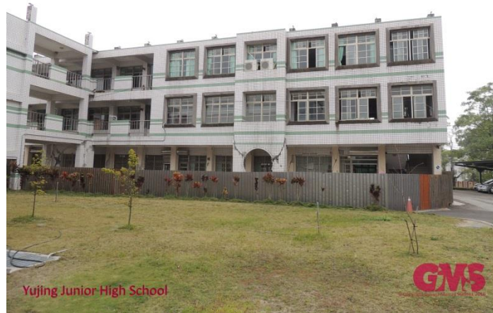
Figure 8: Yujing Junior High School Not Retrofitted (Severely Damage)
