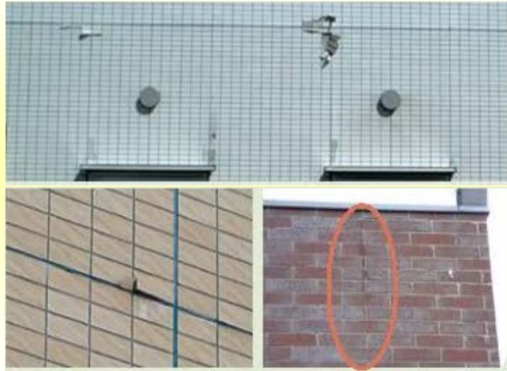
Example of cracking around opening
