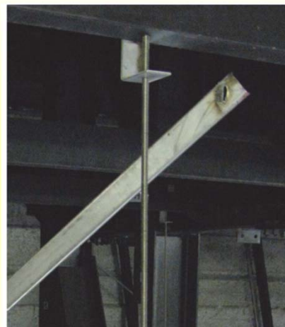
Example of fractured welding part
