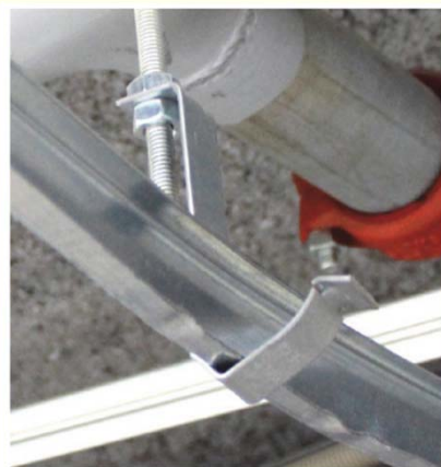
Example of broken hanger
