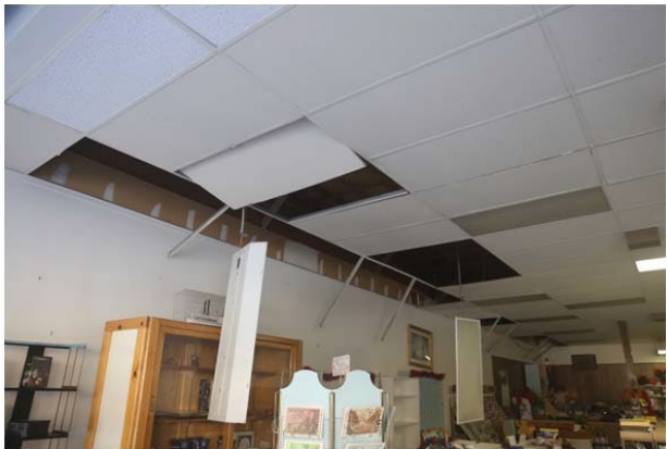
Damage to suspended ceilings
