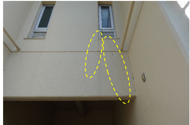
Figure 9. Cracks on RC beam
