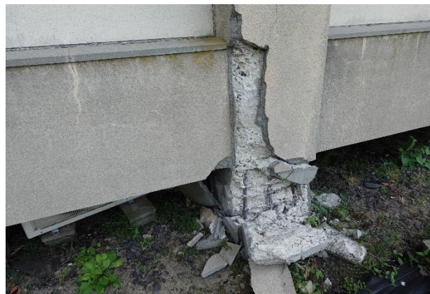
Figure 20. Damage to RC column
