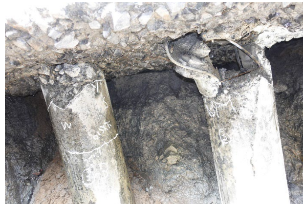
Figure 3. Damage condition of piles
