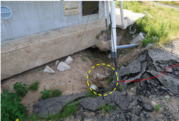
Figure 10. The gap between piles and the upper structure
