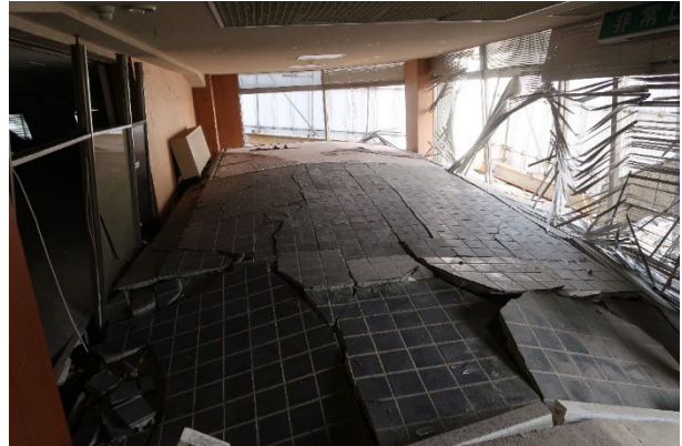
Figure 16. Swelling of the first floor
