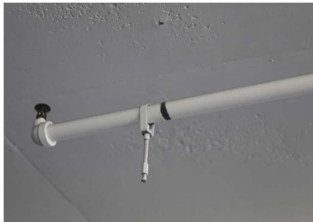
Damage to sprinkler system
