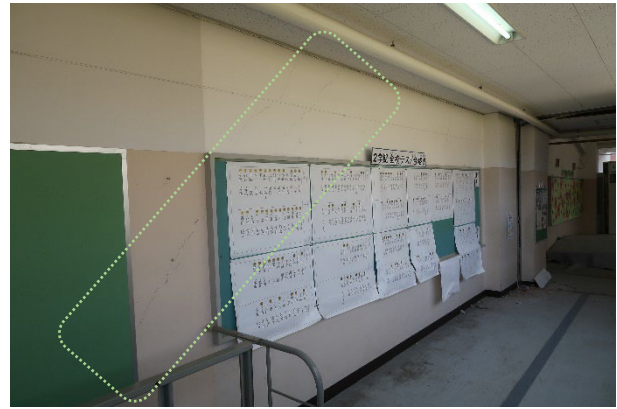
Figure 7. Shear cracking of wall
